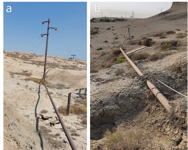
Figure 5. Example of infrastructures built across the creeping mud flow at Lokbatan MV. (a, b) Ongoing flow movement causes deformation of the pipeline.
