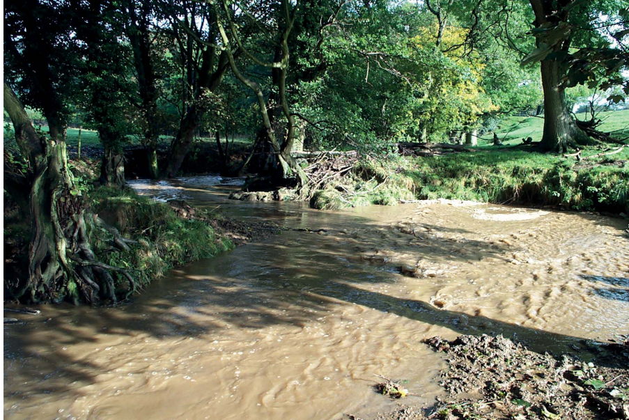
Figure 4. View looking downstream of the channel diversion during the construction phase. Photograph taken on day of diversion works; 10 October 2007.
