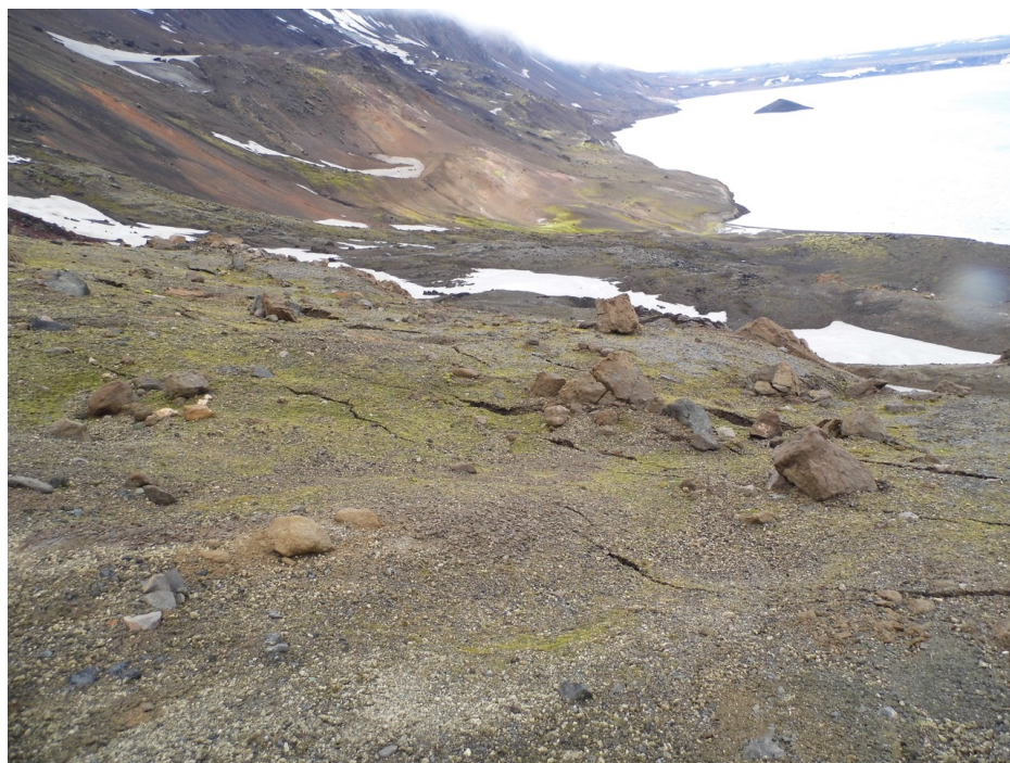
Figure 3: Cracks on top of the landslide body in August 2013, a year before the failure. Location of the image is indicated on Fig. 5, view is to the west. Image taken by Daniele Trippanera.
