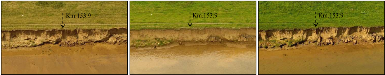
Figure 13: Zoomed-in UAV photos from track 1 at section 4, km. 153.9, showing diverse bank erosion stages: slump blocks at bank toe on June 21 (left), clean bank face after block removal on July 19 (centre), and undermining on August 23 (right).
