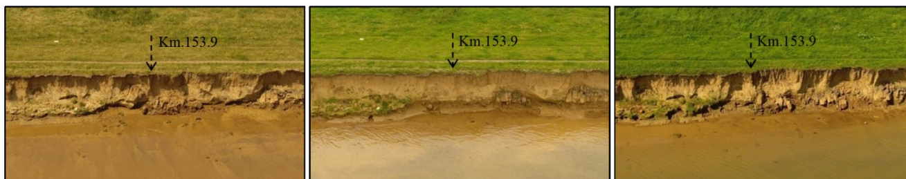
Figure 13: Zoomed-in UAV photos from track 1 at section 4, km. 153.9, showing diverse bank erosion stages: slump blocks at bank toe on June 21 (left), clean bank face after block removal on July 19 (centre), and undermining on August 23 (right).
