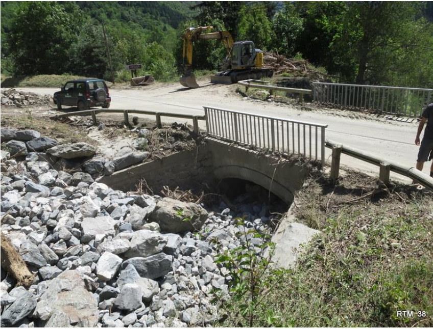
90 Figure 2: Effect of a sediment pulse at a bridge section of the Ruisseau de la Gorge (France), a stream that was known by local engineers for having been inactive for decades. The transported material was much finer ( D_{50} = 96 \text{ mm} , D_{84} = 169 \text{ mm} ) than the bed in place ( D_{50} = 250 \text{ mm} , D_{84} = 413 \text{ mm} ).
