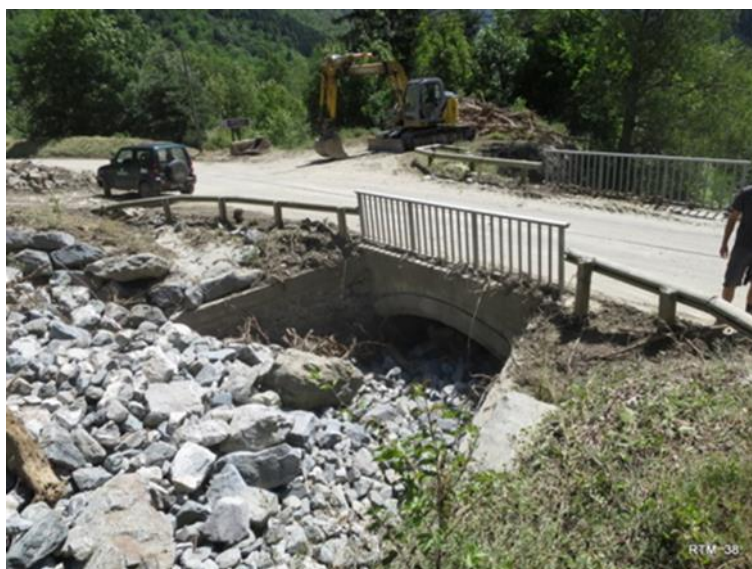
Figure 2: Effect of a sediment pulse at a bridge section of the Gorges river (France), a stream that was known by local engineers for having been inactive for decades. The transported material was much finer ( D_{50} = 96 \text{ mm} , D_{84} = 169 \text{ mm} ) than the bed in place ( D_{50} = 250 \text{ mm} , D_{84} = 413 \text{ mm} ).
